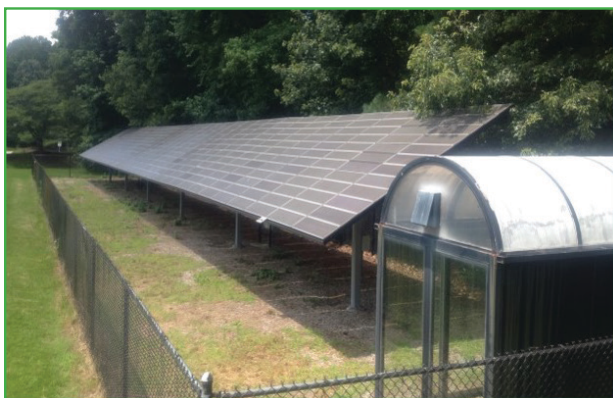
Solar panels at Canon Virginia location.
